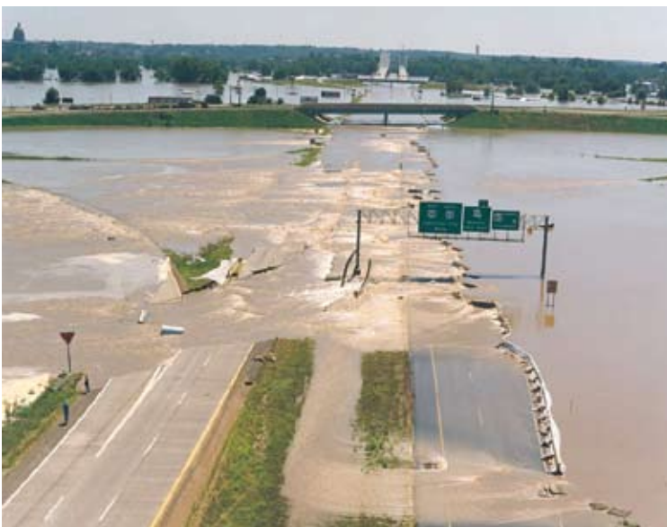
The Great Flood of 1993 caused flooding along 500 miles of the Mississippi and Missouri river systems. The photo shows the flood's effects on U.S. Highway 54, just north of Jefferson City, Missouri.
